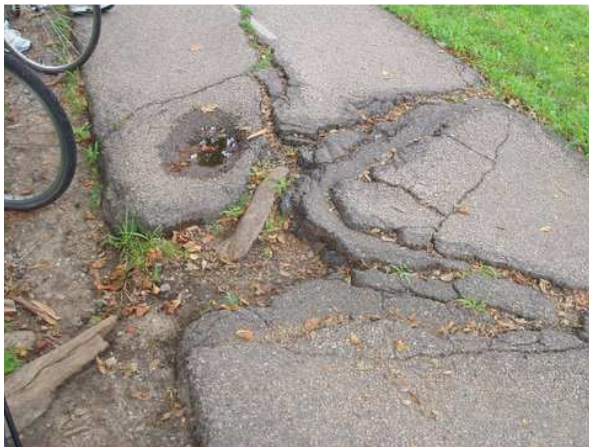
Figure 1 Root Heave, Cambridge, East of Eliot Bridge
