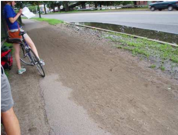
Figure 11 Debris Accumulated on Path, Near Magazine Street, Cambridge
