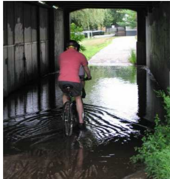
Figure 12 Water and Mud Accumulation, Eliot Bridge, Cambridge
