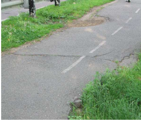
Figure 3 Large Pothole, Cambridge, Across from Hawthorne St.
