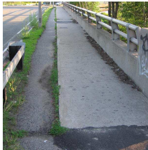
Figure 2 Pavement Differential, Boston, East of Arsenal Street
